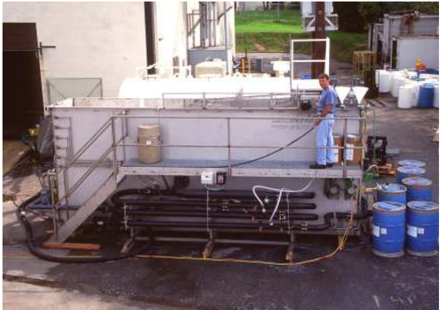
IWWS 0-200 LS PhysicalChemical waste treatment system includes flotation compartment, sludge holding, polymer holding and extended reuse holding along with all pumps on one skid. Setup time was four hours.
