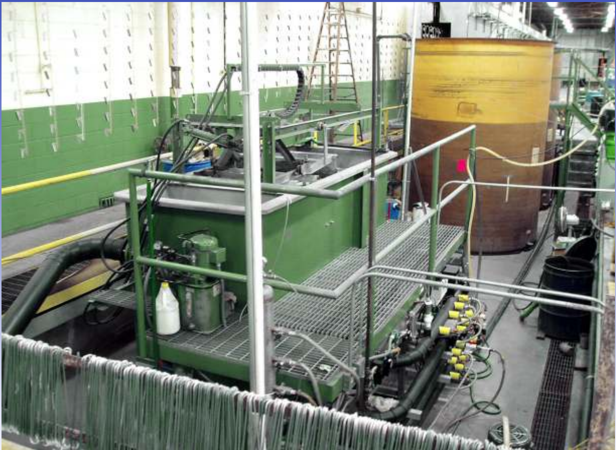
Continuous Metals Removal Waste Treatment System Installed at Royston, LLC replaced a much larger precipitation system that constrained plant operations. IWWS operates the system for the customer and is responsible for compliance.
